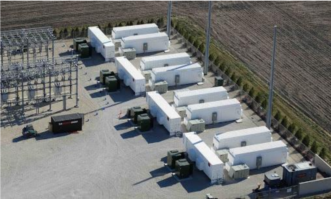
FIGURE 8-7 A STOCK IMAGE OF A SIMILAR DEVELOPMENT WITH AN ON-SITE SUBSTATION AND BESS
