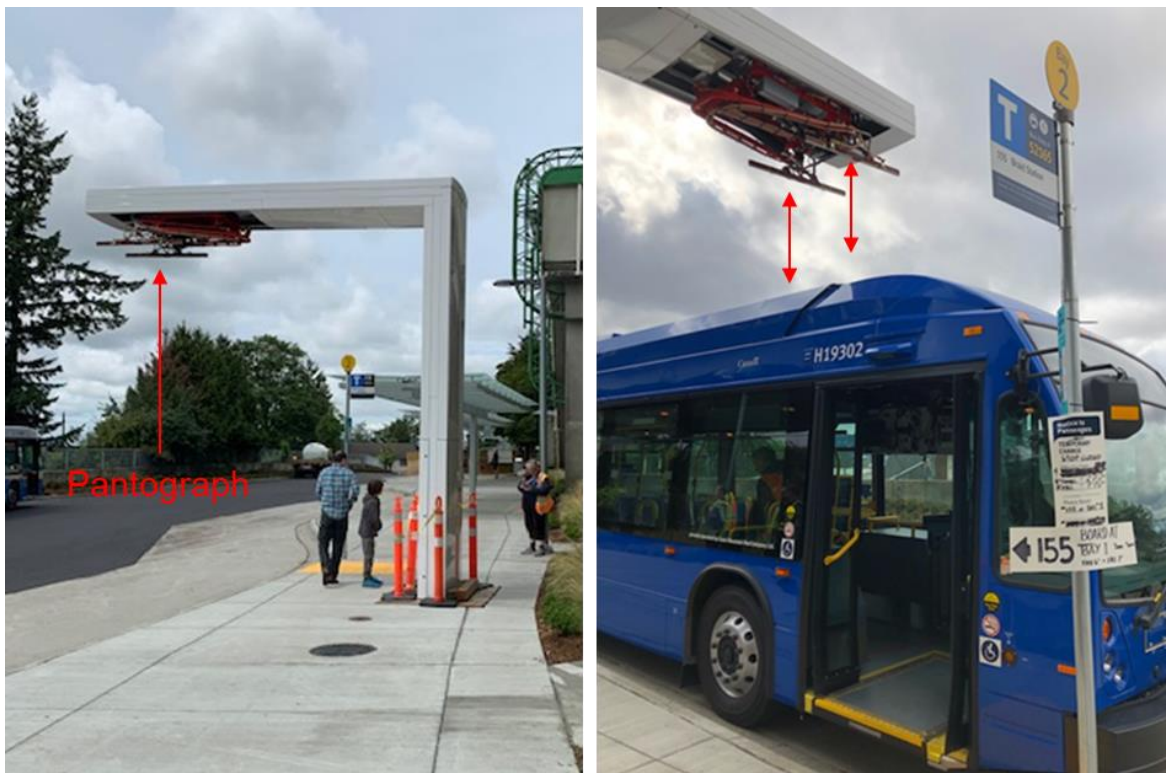
Figure 5 Typical In-route Charger Installation
